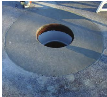
The concrete is poured to the exact grade of the manhole lid and the road.
